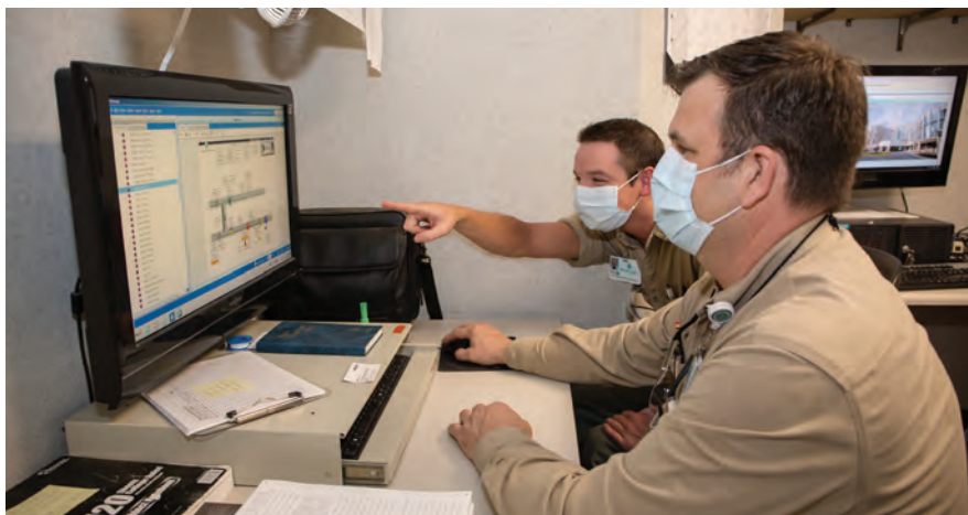
Jody Hensley (foreground), mechanic four, shows Tyler Roper, mechanic two, how to adjust fan speeds and valves to maintain patient comfort while saving energy on the hospital's building automation system computer.
