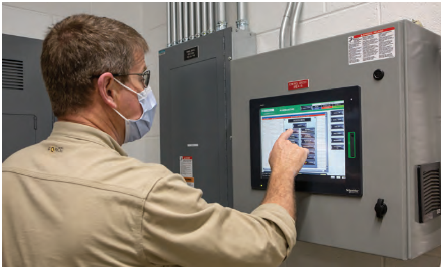
Ronald Morehead, mechanic four and lead electrician, checks power consumption rates on the main switchgear for the hospital's energy plant.
